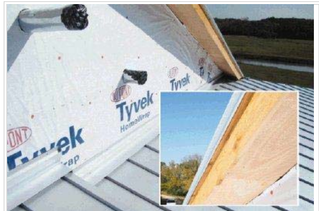
All flashing is provided and installed by the roofer before the final cladding is applied to the house (brick, siding, stucco, etc.)
